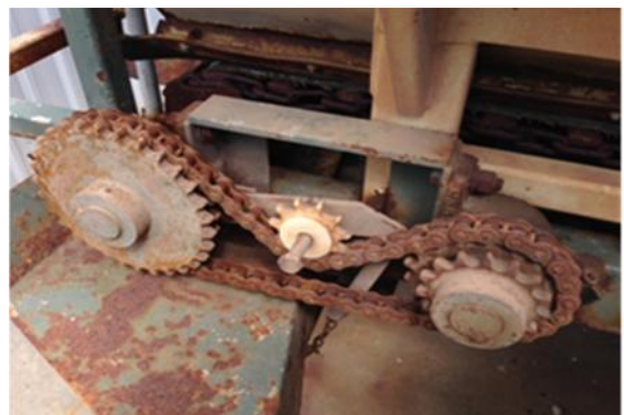
Chain guard missing
